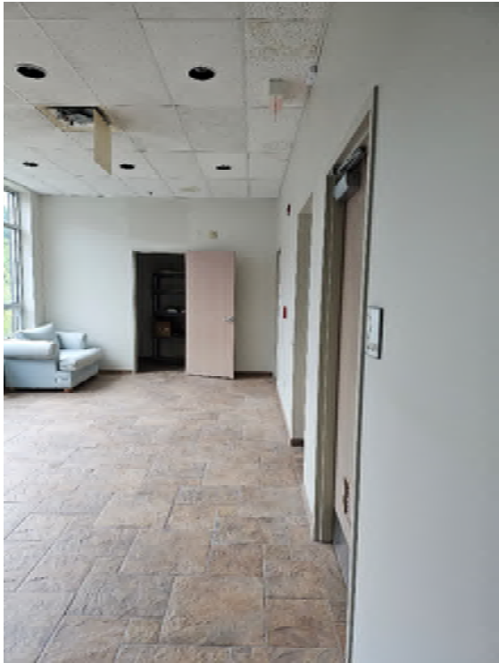
Figure 6 Exit sign is not visible from path of travel
