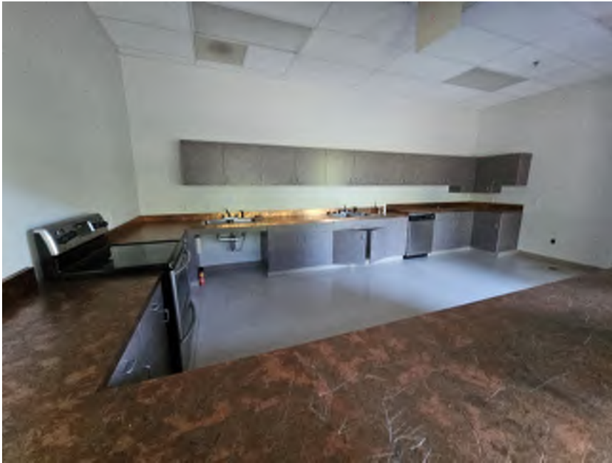
Figure 1 Main Kitchen at Breakroom: No range hood, no pipe insulation under sink(
