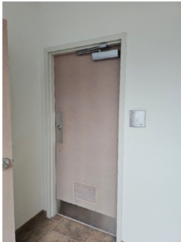
Figure 4 Added wall encroaches on ADA clearance into restroom (4 occurrences)
