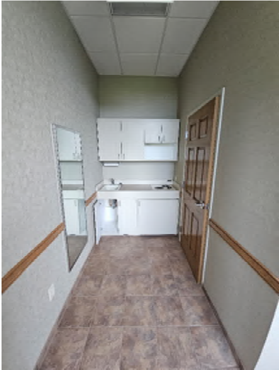
Figure 5 Kitchennettes are not accessible and no hood over burners.
